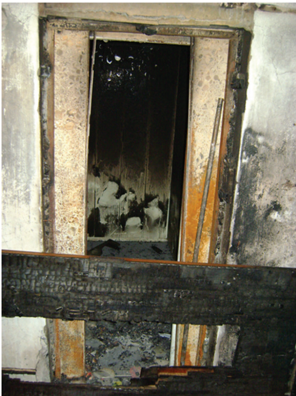
Figure-3: Tarangan CHS Elevator (post incident)
